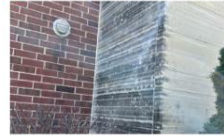
1 Damaged/Discolored Limestone Panel
