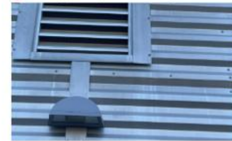
13 Damaged/Dirty MTL Wall Siding
