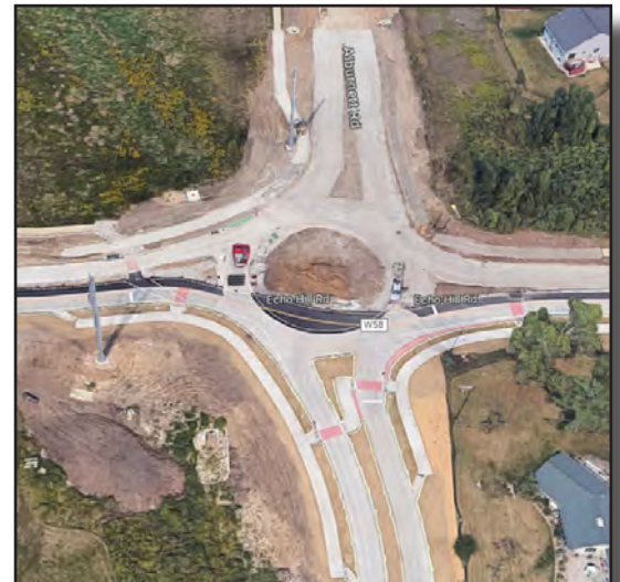
Construction of the roundabout at Echo Hill Road and Alburnett Road. It opened in the fall of 2022.
