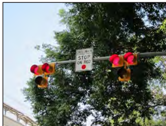
Image 35: Example of a pedestrian hybrid beacon on a stop light arm mast. Source: Federal Highway Administration
