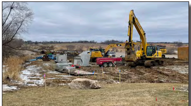
Grading and utilities construction on Tower Terrace Road between Alburnett Road and C Avenue in Cedar Rapids.
