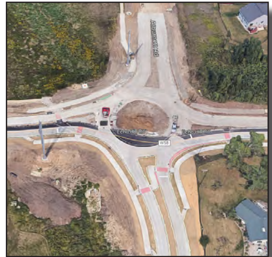
Image 38: Constructing the roundabout at Echo Hill Road and Alburnett Road. It opened in the fall of 2022.
